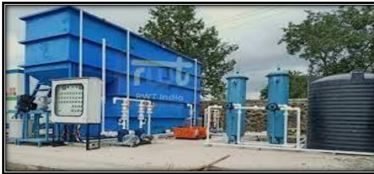
Fig 4.1 Sewage treatment plant [Source: - KPA Web]
