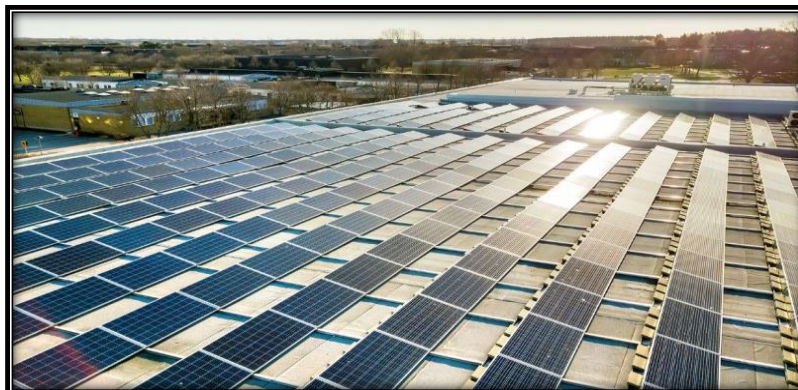
Fig 4.2 200-MW of Rooftop Solar Systems [Source: - Mormugao Port Authority Web]
