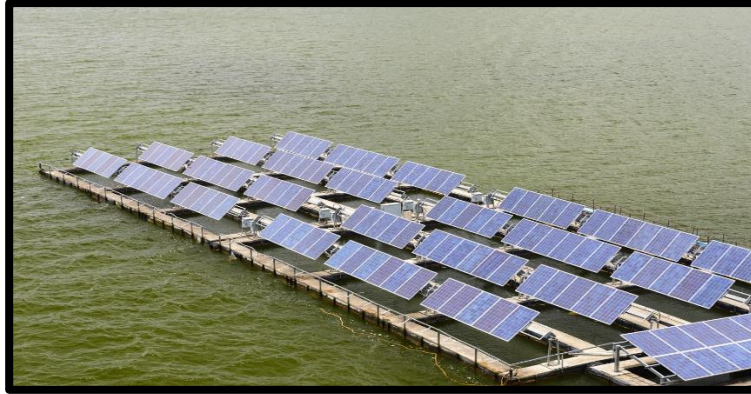
Fig 4.4 Floating solar plant at Cochin Port [Source: - Cochin Port Authority Web]
