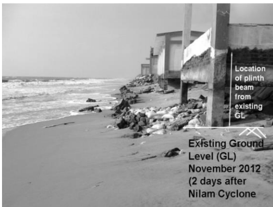
(a) Erosion after 'Nilam' cyclone November 2012
