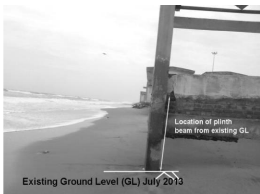
(c) Erosion as of July 2013 (tilt of column is due to image orientation)
