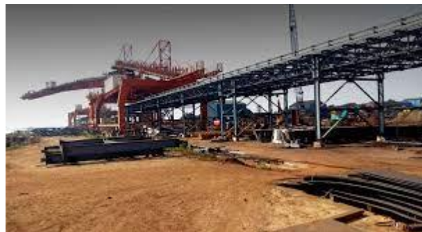
JSW Infrastructure of Iron Ore Berth
