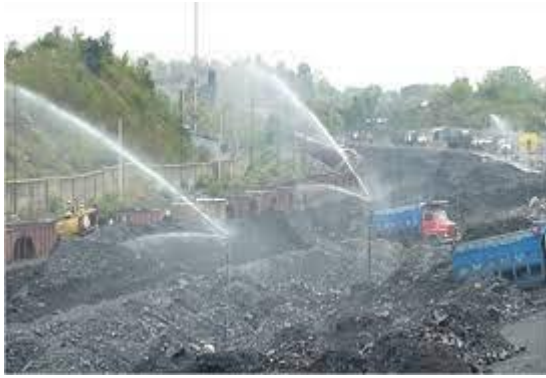
Dust Suppression System
